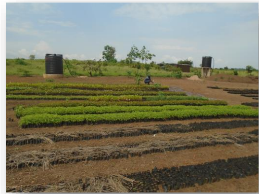
The new solar irrigation system
